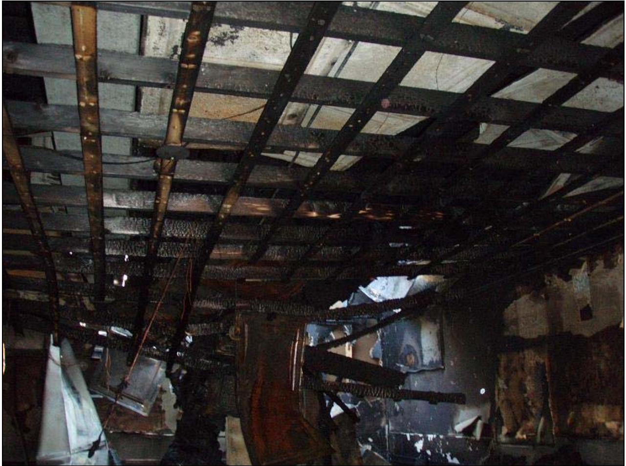
Photo 6. View looking towards kitchen and D-Side wall from dining room at exposed furring strips where the ceiling tiles were attached prior to the rapid fire event. (Photo courtesy of fire department.)
